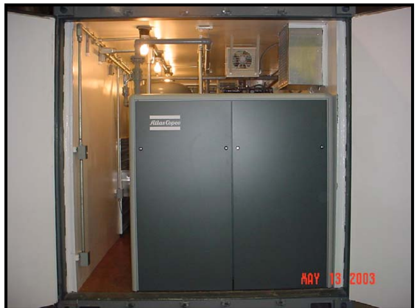
GreenPort Power Project In an outdoor container
